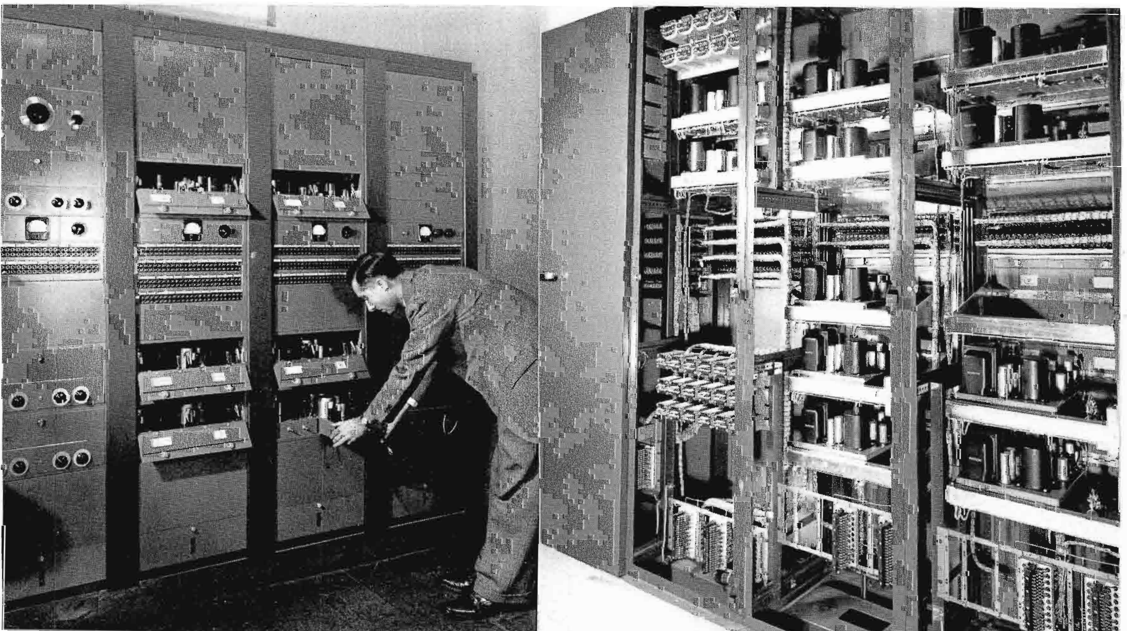
FIG. 4. Rear view of three Master Control audio equipment racks with doors removed to show neat mechanical design and orderly arrangement of parts. Note how all wiring is carefully "dressed" and brought out to terminal strips.
